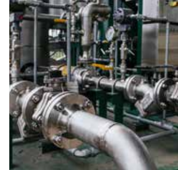
BOILERS AND BLOWERS
